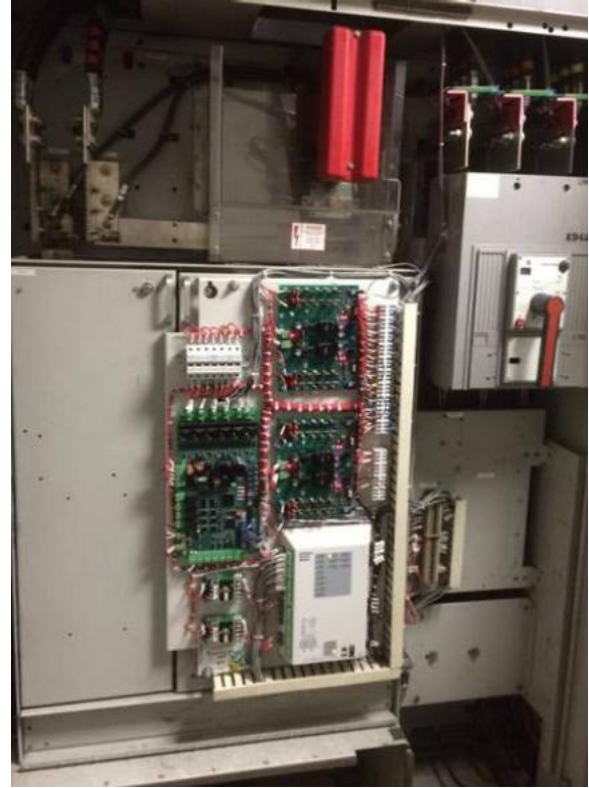
Fig. 14 New control electronics with existing power bridges
