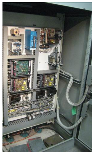
Figure 1. The original VR 45 voltage regulators, transducers, power supplies, and PT/CT test switches
