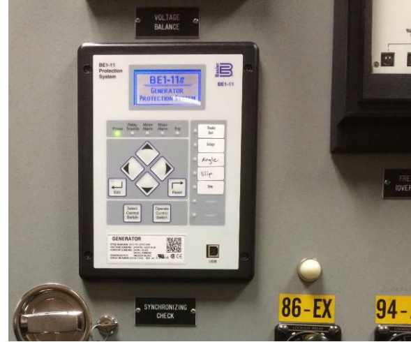
Figure 8. The BE1-11g Generator Protection System
