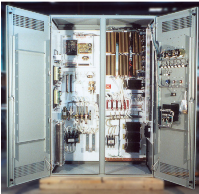
Figure 1. Basler Electric SSE Cubicle
