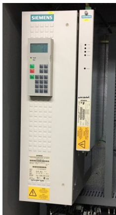
Figure 1 - Siemens RG3 Voltage Regulator
