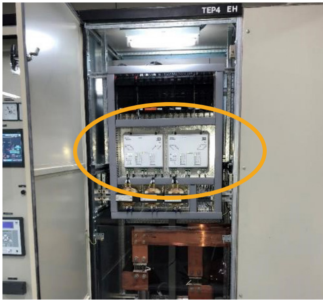
Figure 6. IT-2 transducers for measuring the excitation transformer voltage
