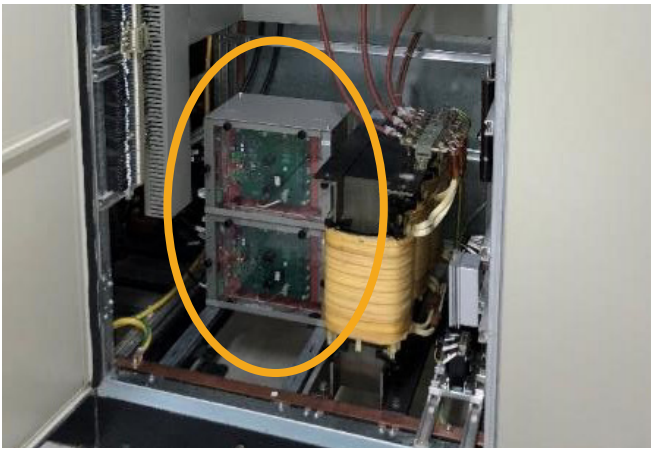
Figure 9. DXCB-2 modules (field discharge)
