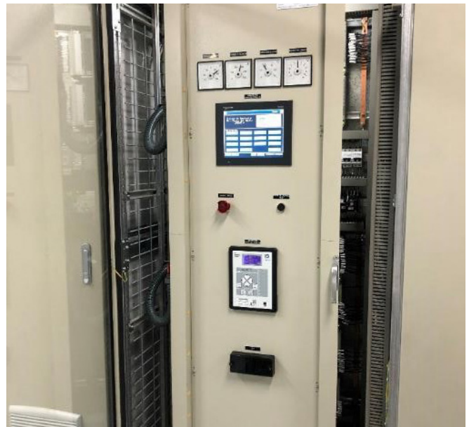
Figure 8. New front end of the cabinet with BEI-11r protection relay
