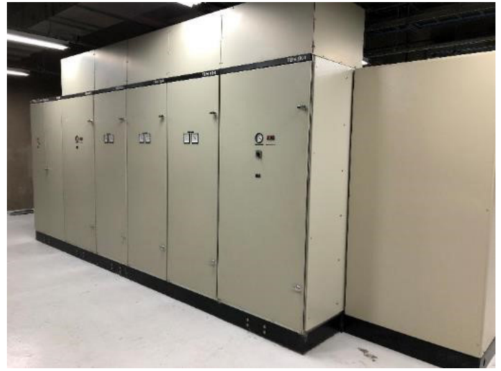
Figure 10. Rectifier Bridges / Cooling System
