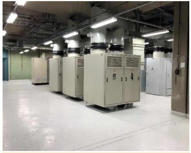
Figure 7. Excitation Transformer Bank (3 x 1,300 kVA - 15,750 kV / 1,120 V)
