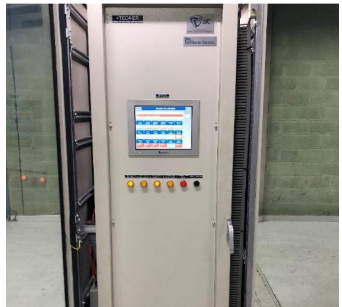
Figure 11. Excitation system's HMI
