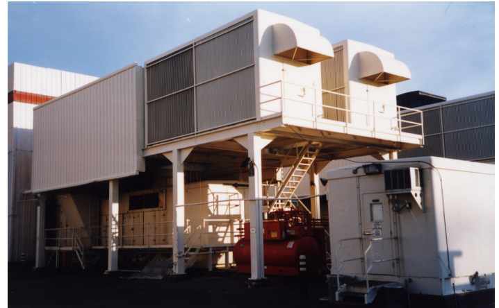
Figure 3. Facilities with gas turbines requiring power system stabilizers benefit from negative field forcing voltage regulators.
