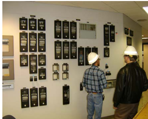
Fig. 4 Old EM Transformer-Differential Relays
