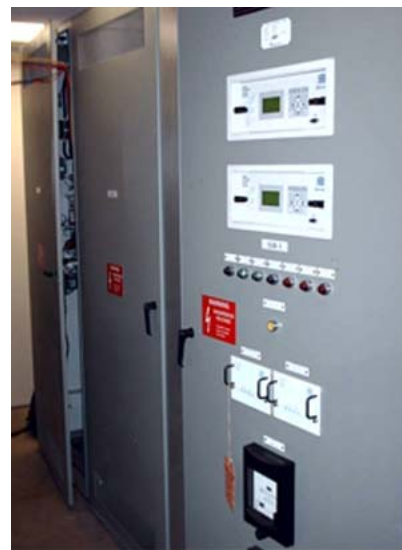
Figure 9. Cabinet with Redundant Digital Excitation Control Systems
