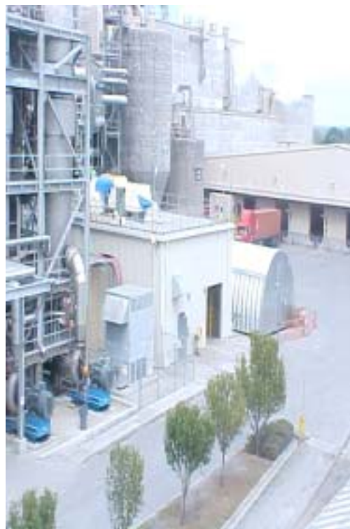
Fig. 1: New Turbine Generator and Reactor installed at the Recovery and Utility Complex
