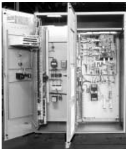
Figure 6: Excitation cabinet installed in the new Generator EER
