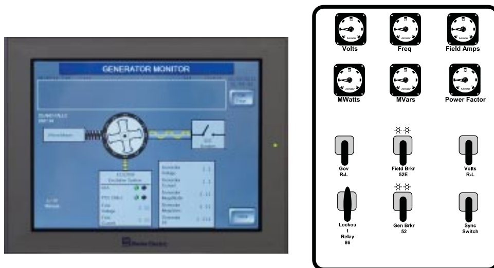
Figure 27: Common Remote or Local Controls
