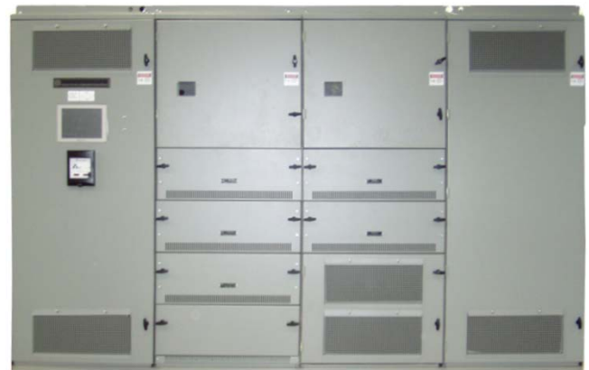
Fig. 10. New Static Exciter with Power Rectifier Drawers, with local HMI for Metering and Alarm Information
