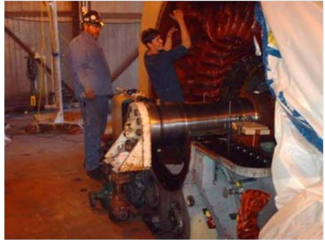
Fig. 6 Brushless Exciter Removed from End of Shaft
