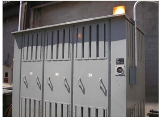
Fig. 9. Power Potential Transformer
