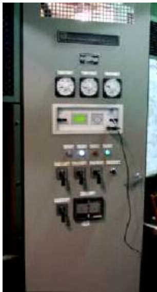
Figure 13: New front door provided with new cutouts for DECS-400, a serial cable is used for a laptop connection.
