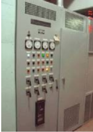
Figure 12: Using the analog technology; many lights, switches and meters on front of doors of a Basler SSE Static Exciter
