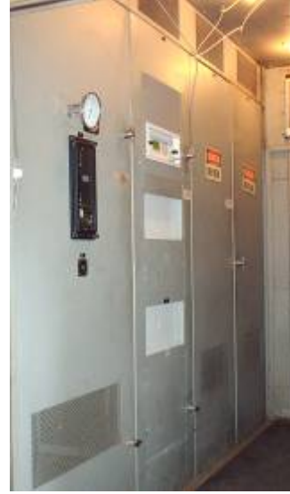
Figure 6: Exciter cabinet lineup with DECS-400 installed
