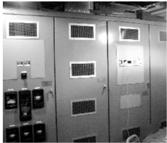
Figure 14: The Lineup of the Siemens Allis Original Equipment; The DECS-400 digital controller installed on front of Siemens Allis Cabinet. Metering and obsolete switches were removed.
