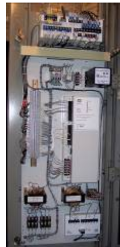
Figure 5: Back door of DECS-400 panel showing IFM Firing Circuit and related hardware
