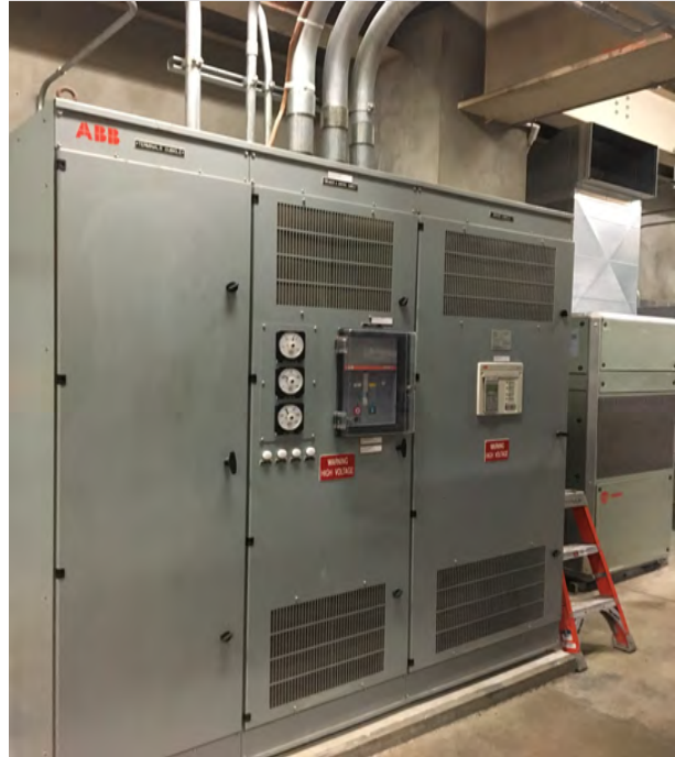
Unitrol F static excitation system (before)
